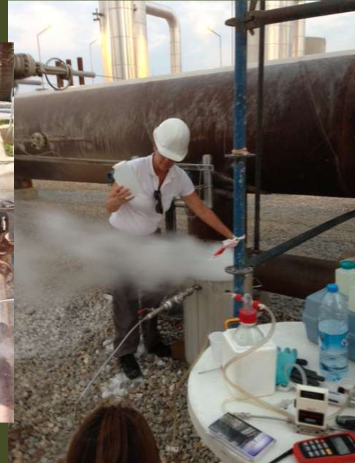
Kizildere II, Turkey, Plant Inlet
